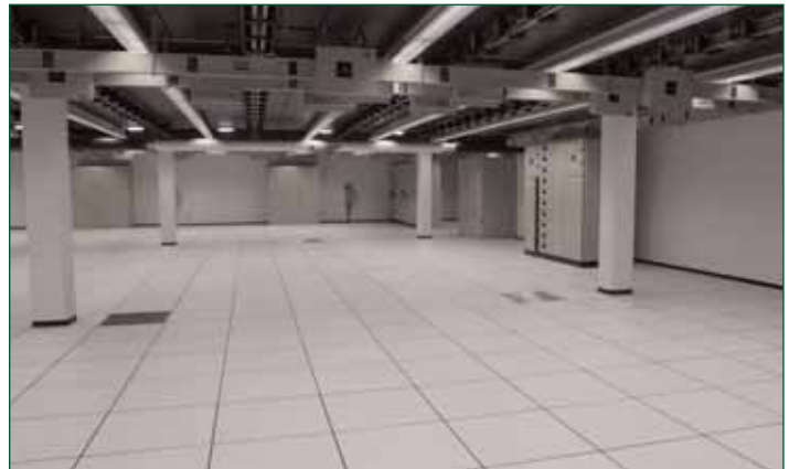
Typical Conditioned Module Space
